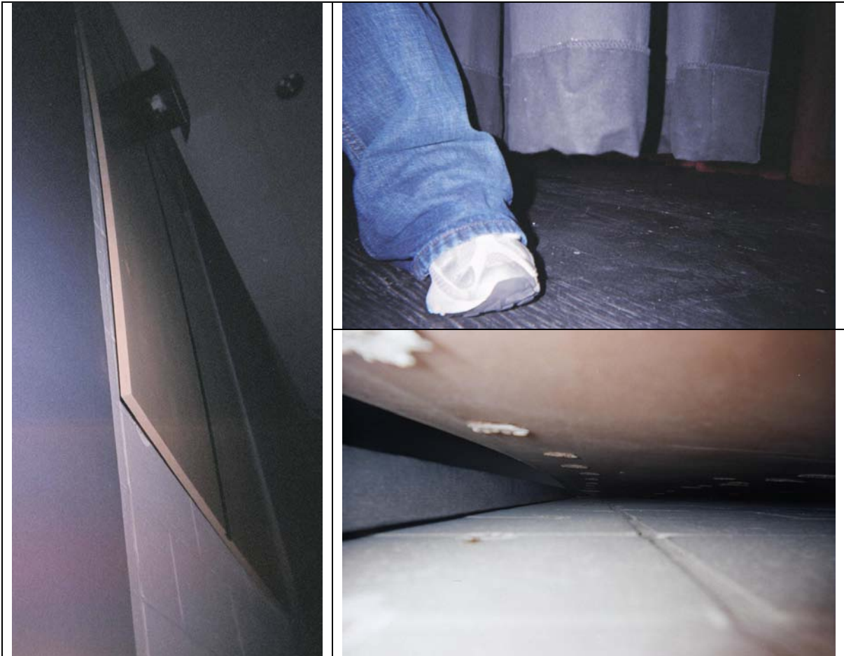
Figure 2.1: Moisture Damage in the Auditorium. Left: Warped wooden paneling. Top Right: 6" shrinkage of the building curtain. Bottom Right: Underside of the wood panel pulling back from the wall.
