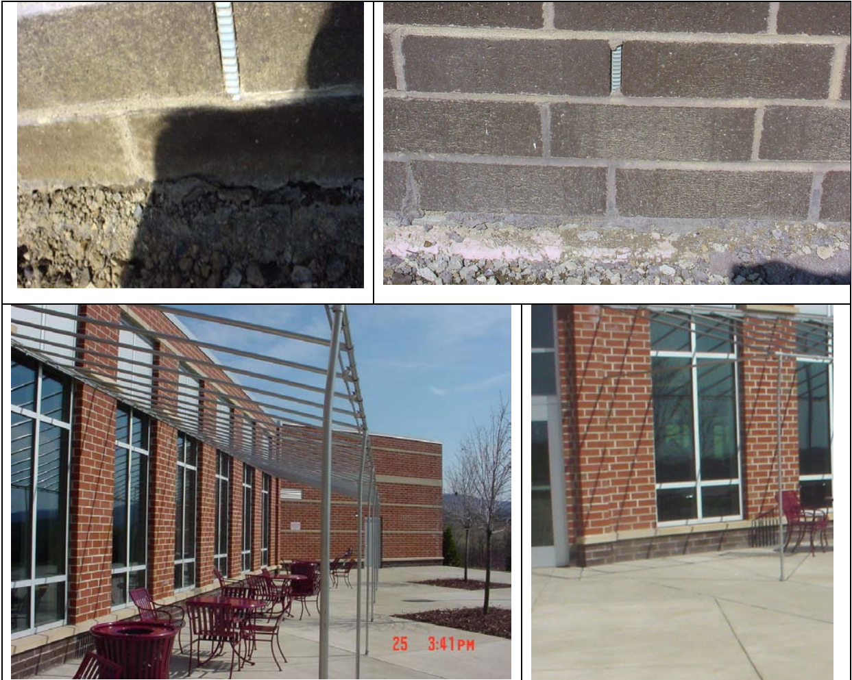
Figure 3.1: Existing Wall Conditions Top Images: Weep Hole in the Correct Location. Lower Images: Concrete Slab to Brick Wall Connections
